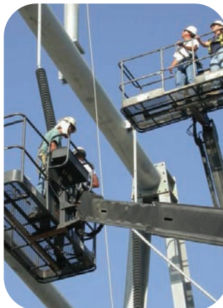
Photo Provided by Southern California Edison
