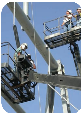
Photo Provided by Southern California Edison
